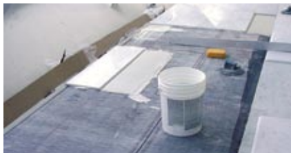
Carrera marble being set over ECB at the Calatrava Expansion of the Milwaukee Art Museum
